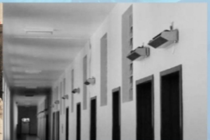
UVGI Upper Room in Naturally Ventilated Corridor of TB Facility in Brazil
